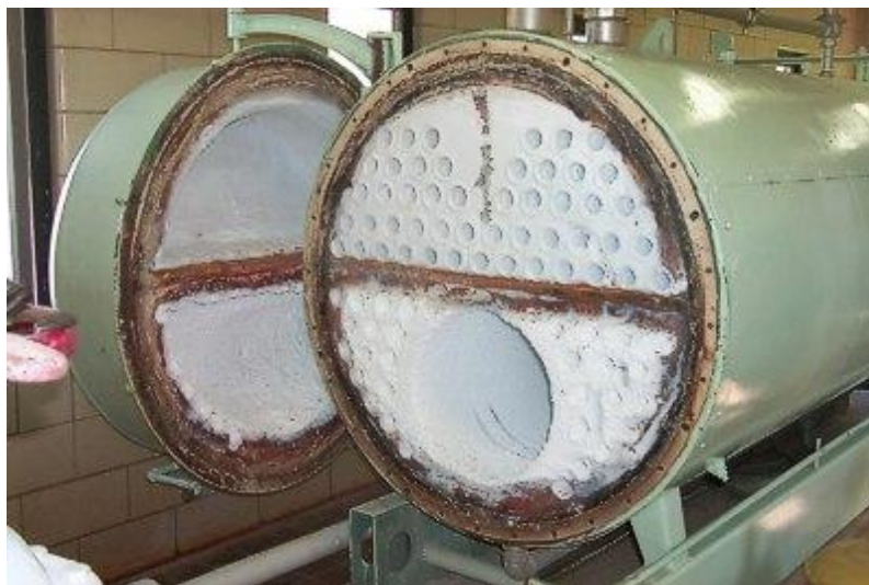
Figure 4. Siloxane Damage to Boiler Tubes
